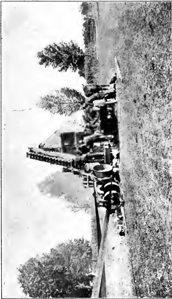
Arrangement of Crushing Equipment—Inferior method of feeding field stone, being hauled one by one to Crusher, while team is idle.
